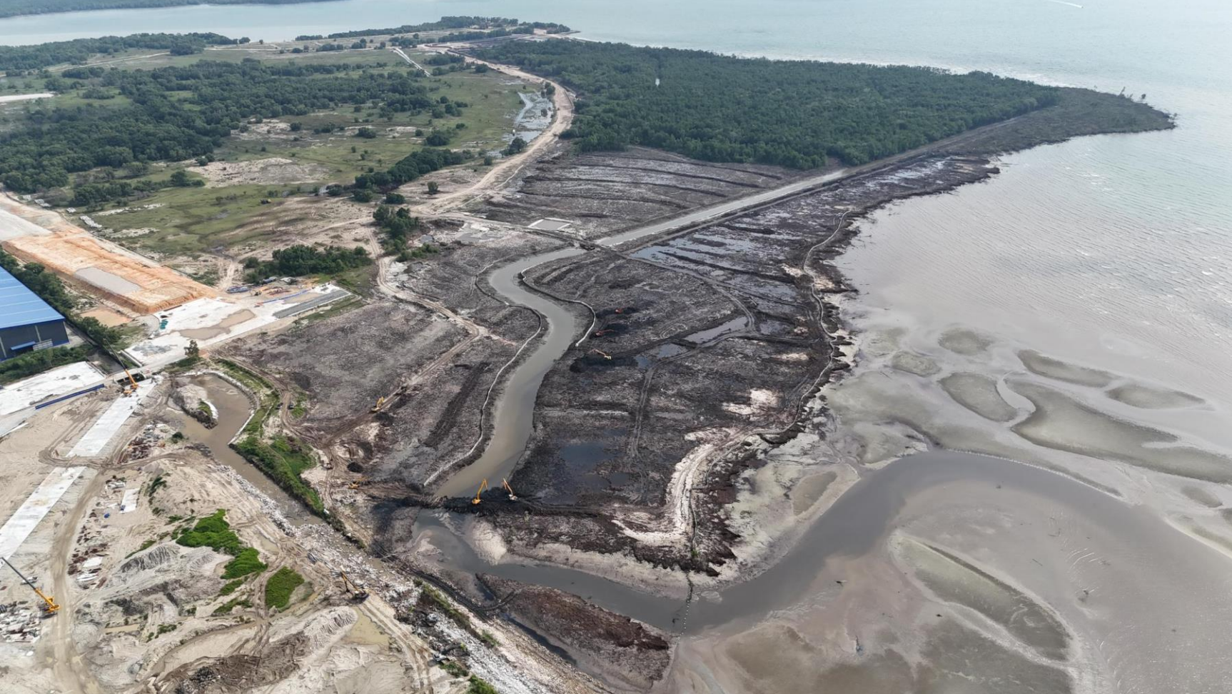
The view of site clearance at Marina Land for the upcoming reclamation work. Actual work progress as of 31 st December 2024
